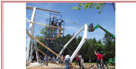
The frame for New York State's first-ever passive house is raised on Millbrook Road in Claverack. (Francesca Olsen/Hudson-Catskill Newspapers)
